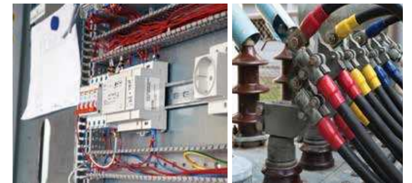
Execution of electrical works and control cables at Tabuk Cement Company factory
